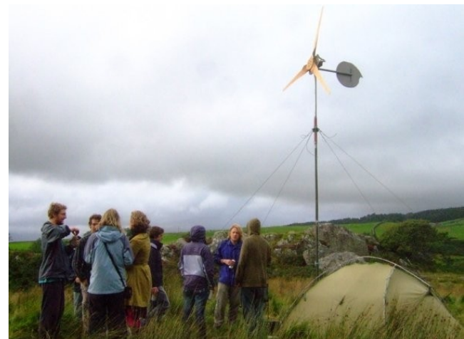
A completed wind turbine in action
